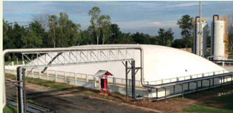
Biogas holder, part of the electricity generation system of Thai Beverage Energy Co., Ltd. in Buriram province
