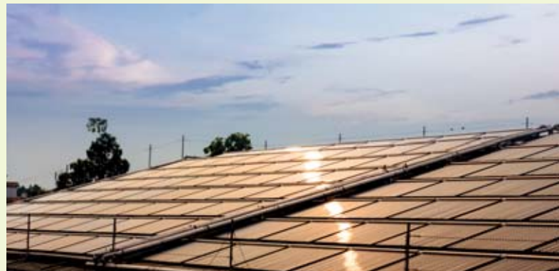
Solar Roof at Sermsuk Public Company Limited
