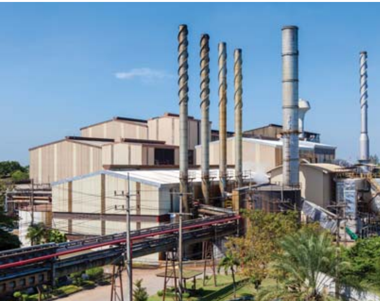
Boiler stacks of our facility at Sura Bangyikhan Co., Ltd.
