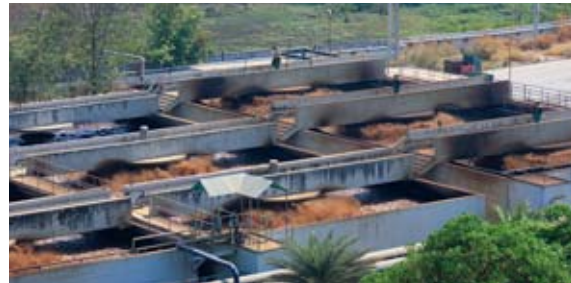
Aerated ponds of wastewater treatment system
